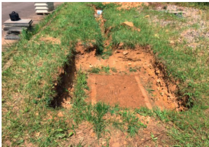
1. After excavating the construction pit, a level, load-bearing and seepage-capable foundation pit base must be created, taking into account the soil conditions.
